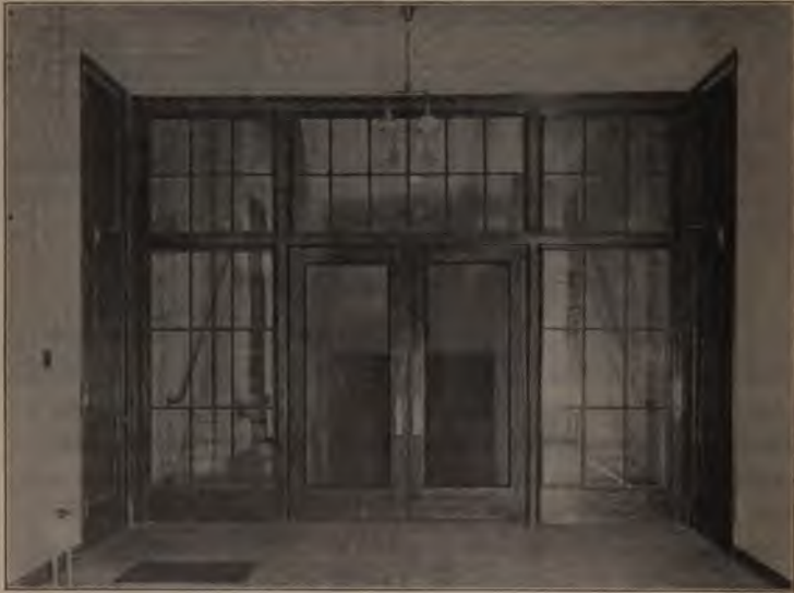
Example of fireproof "smoke partitions," between stairways and corridors, required by the Ohio Code.
